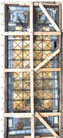
Large stain glass window 12' 1/4 x 56 3/4" w Condition, as is, needs restoration, missing glass, cracked glass, frame in poor condition PreSale Estimate: 500.00 - 700.00
